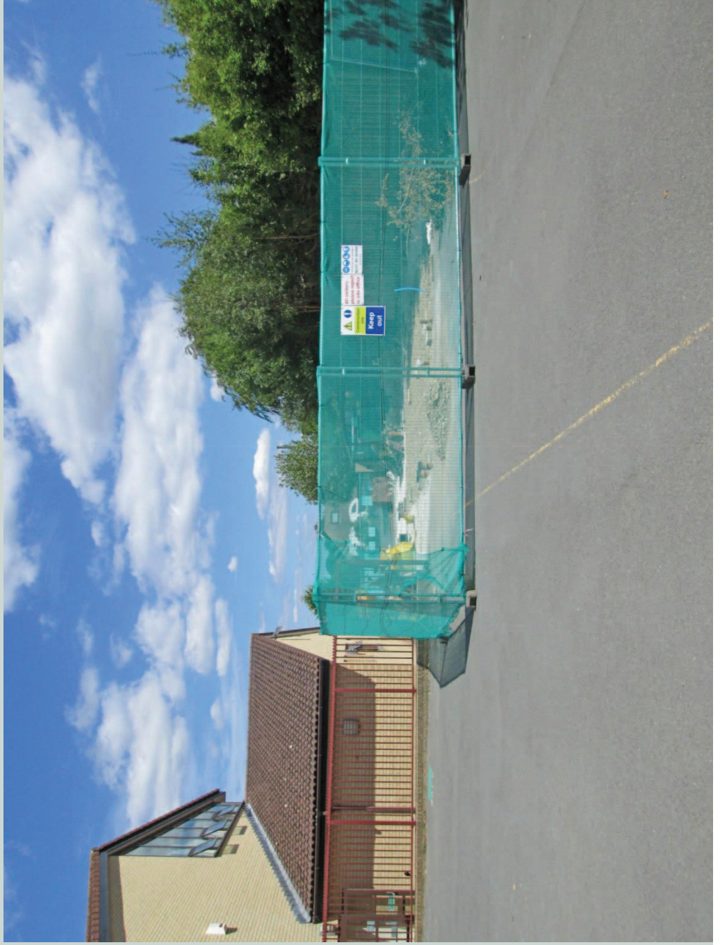
Fig 2 : View looking north from hard play area toward location of demountable unit
