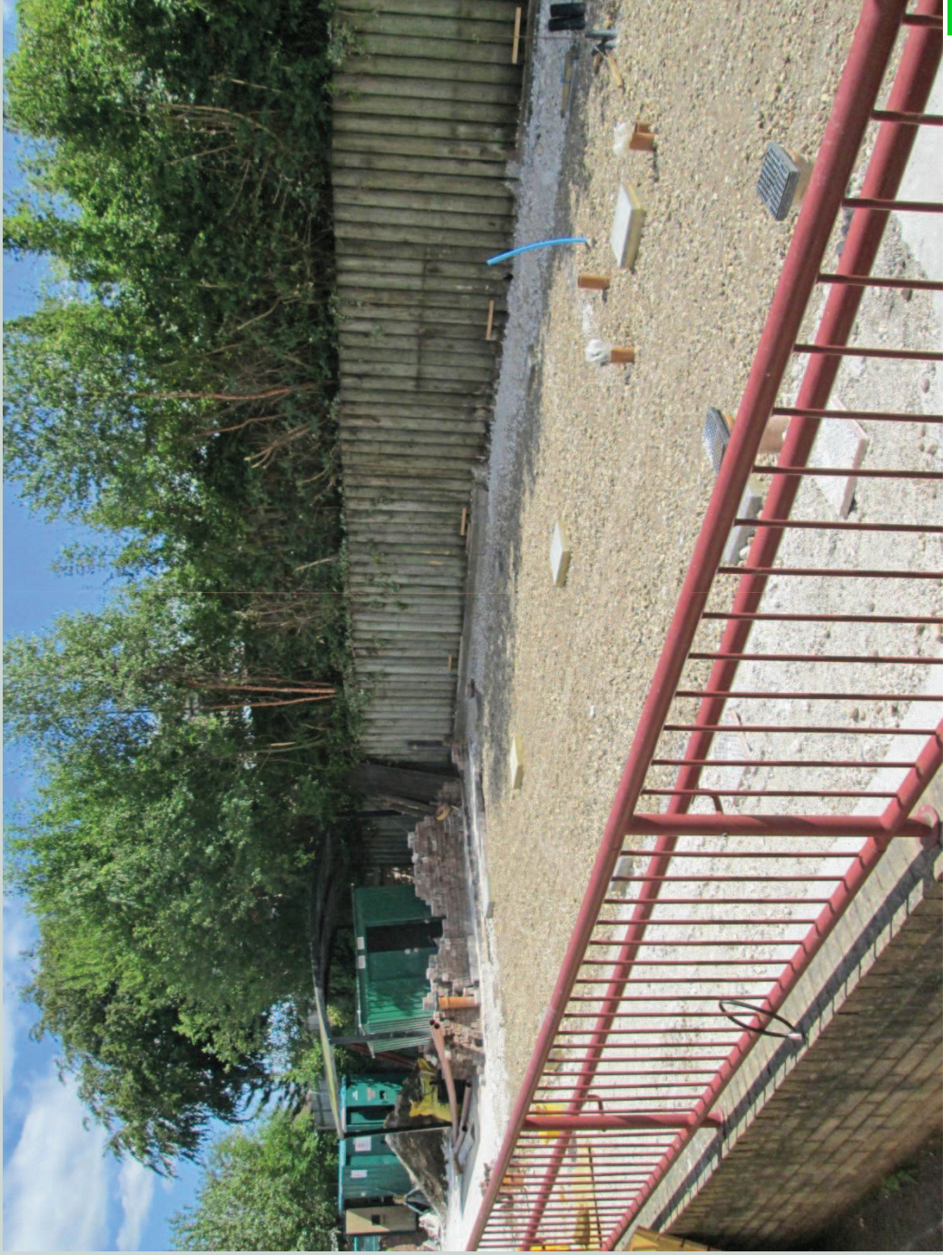
Fig 3 : Looking northeast toward location of the demountable unit, with footings in place
